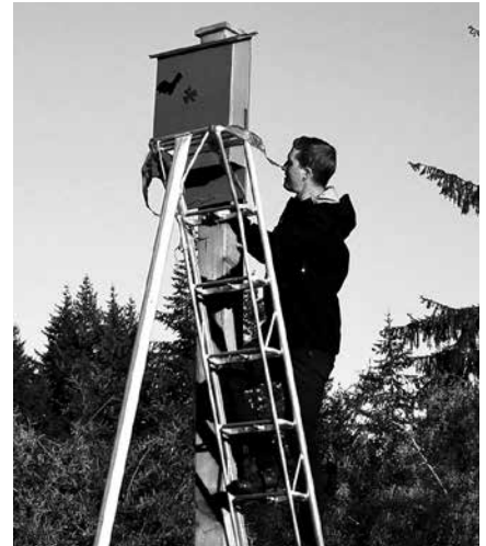
Brad Parrish from the City of Coquitlam, installing the Guides’ finished bat house at Mundy Park. Photo: Audrey Wang
